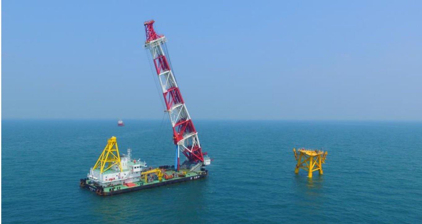
Anemometer Tower Installation Project for Offshore Wind Power in Nan'ao Island, Shantou, Guangdong
