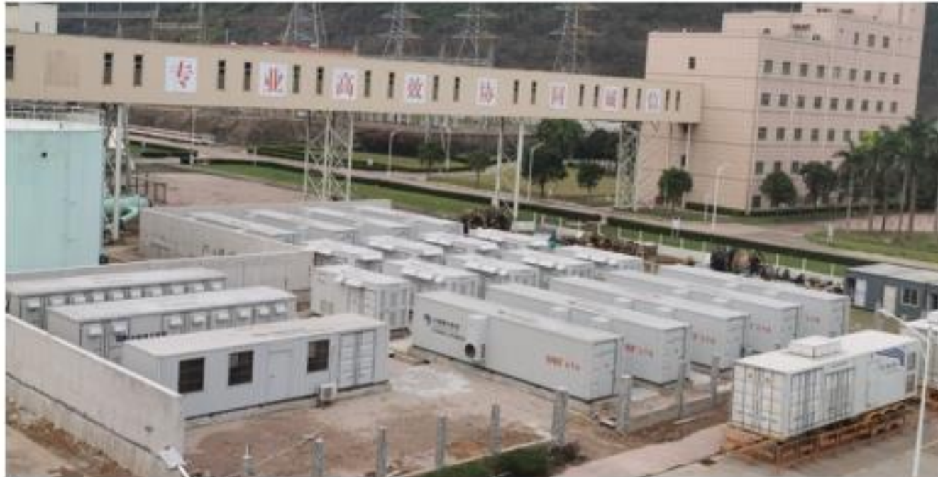
Guangdong Electric Zhuhai power plant energy storage power station project
